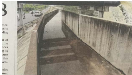
A long concrete wall built to protect Bang Pa-in Industrial Estate in Ayutthaya from possible floods. CHANAT KATANYU
